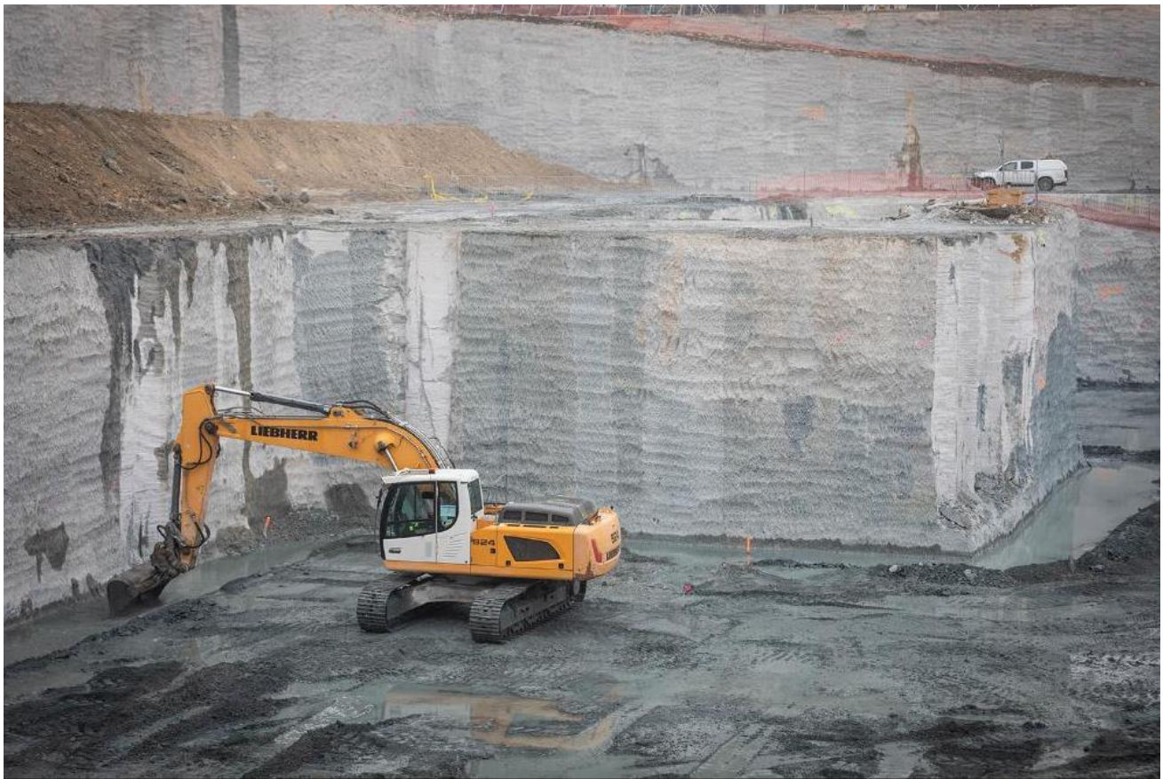
The construction site of the Paks II Nuclear Power Plant, nuclear island of Unit 5 in the location of the lower part of the Southern working pit affected by collapse (The photo was taken by Paks II. Ltd.)
